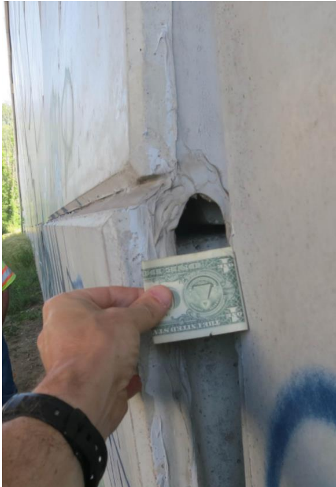
Relative movement of concrete panels
